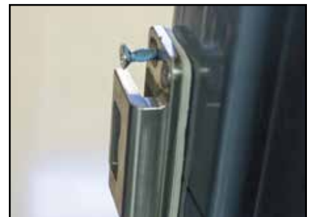
18i & j - Apply Thread Locker to strike screws and attach strike. Remove the (2) previously installed screws, apply Thread Locker and re-install
